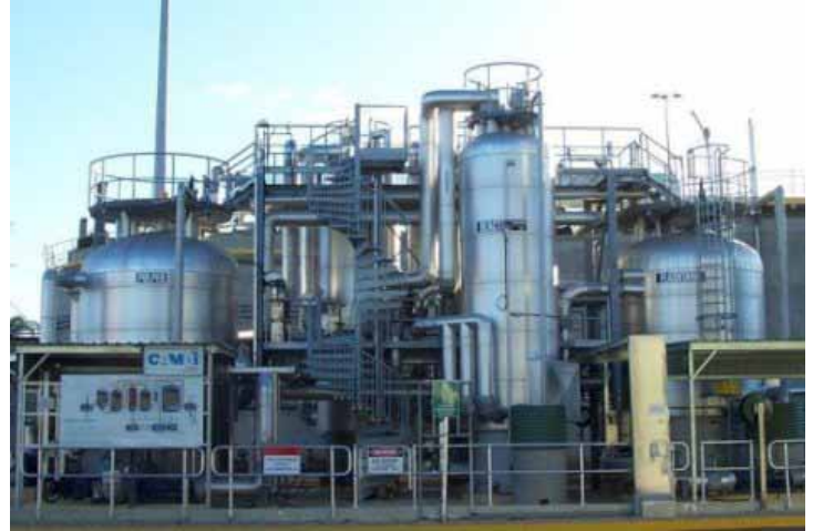
Above: An Anaerobic Digester plant!
